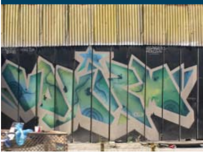
Existing graffiti to be removed
